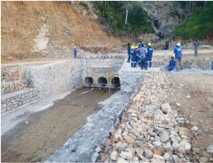
Figure 7.1: Concerns over perceived poor workmanship and materials
