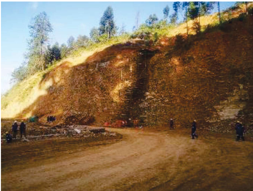
Figure 7.2: Rocks still falling off road cliffs and bridges
