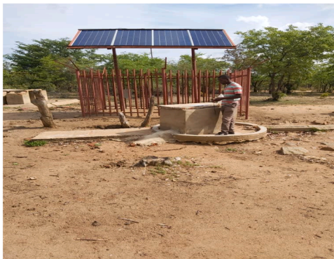
Plate 3. Solar pump installed at a borehole in ward 10 Mwenezi District.
